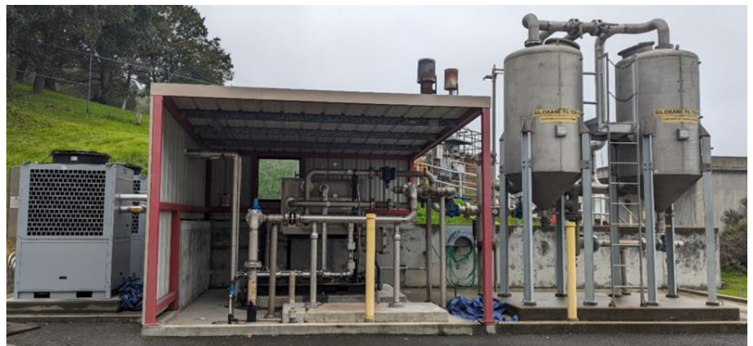
New chillers and heat exchanger for biogas treatment system in service
